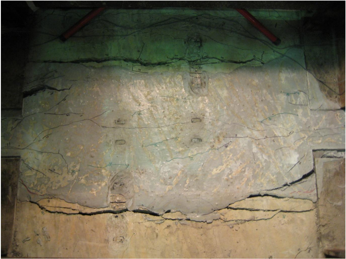
Figure 4.59. Bottom-of-Deck at Failure
